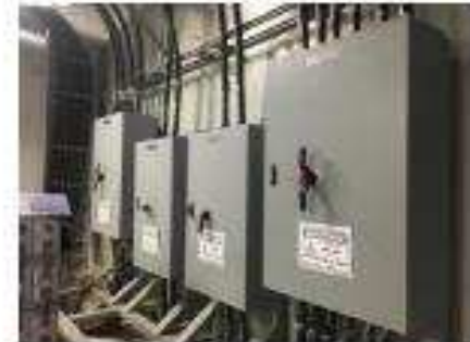
DC disconnecting SW
