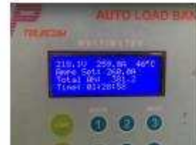
Discharge the 2.600AH Energsys battery bank
