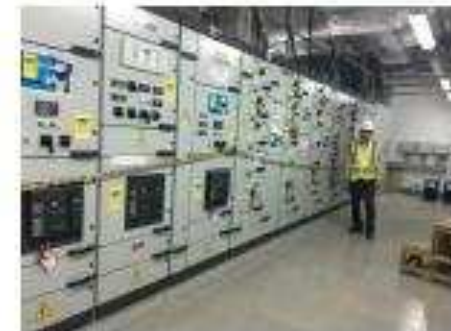
UPS/ DC Power supply
