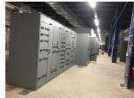
UPS/DC Power supply
