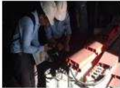
SAFT Battery bank
