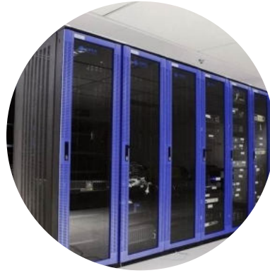
BMS of Telecom
